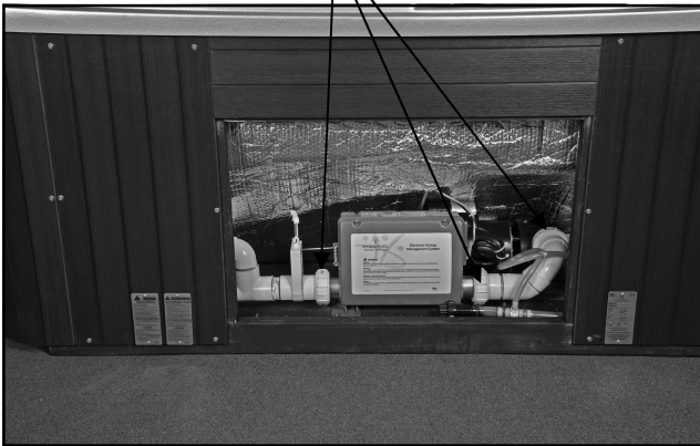
...THROUGH THE PUMP UNION
